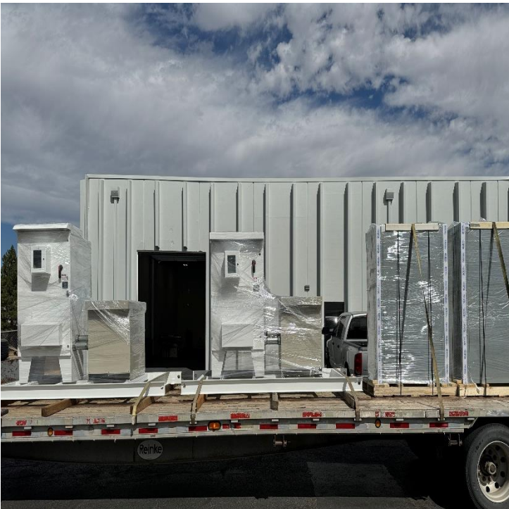
Twin 250 HP VFDs with Sine Wave Filters
